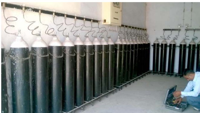
Gas Manifold with Control Panel
