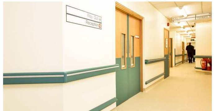
Wall Protection Hand Rail
